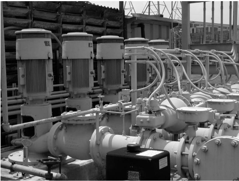
Figure 6.22 Maintenance and repair is a significant component of pumping system life-cycle costs, and an effective maintenance program can minimize these costs. (Courtesy of, and with joint permission of the Hydraulic Institute, Parsippany, NJ; Europump, Brussels, Belgium; and the U.S. Department of Energy Office of Industrial Technologies, Washington, D.C.)
